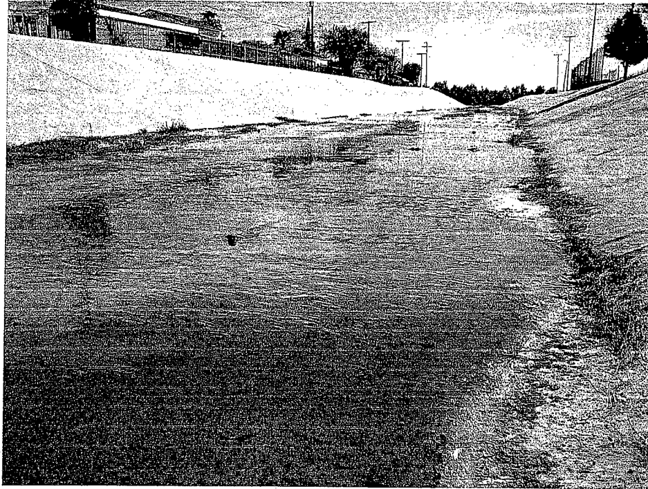
Figure 5: Santa Anita Wash inlet.
